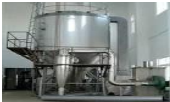
Fig. No. 4: Spray dryer
